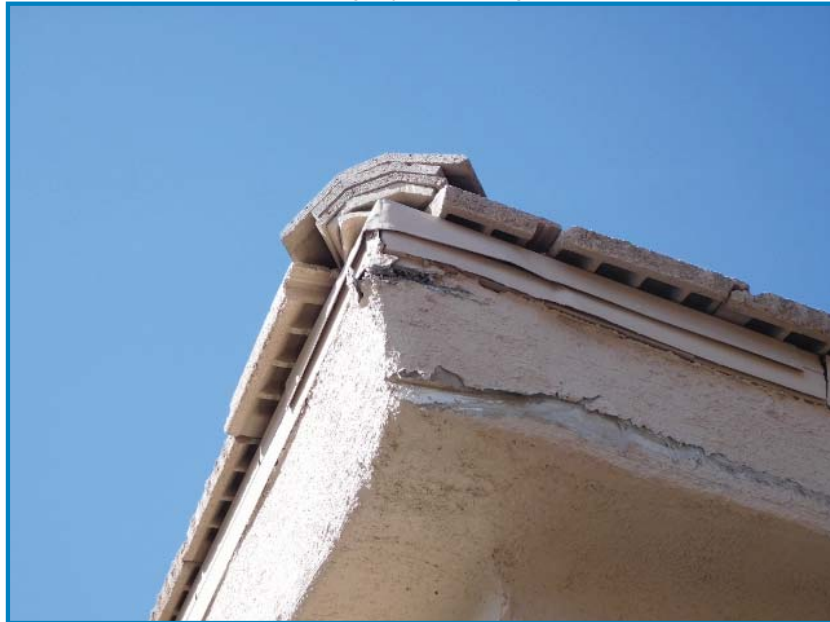
Damage to gatehouse header at entryway
