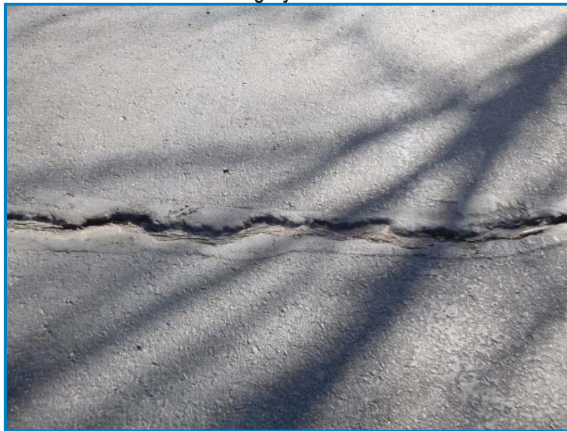
Typical asphalt cracking
